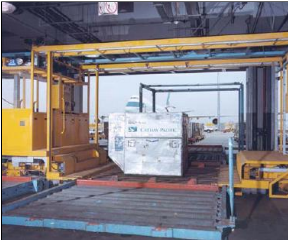
Figure 2.12 Loading ramp facilities ( Siemens 2006 )
